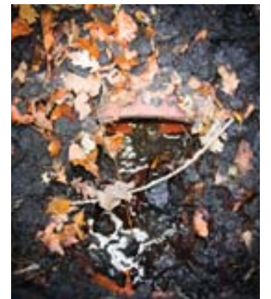
A clogged drainage pipe
